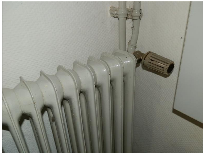
Thermostatventil, stark veraltet
